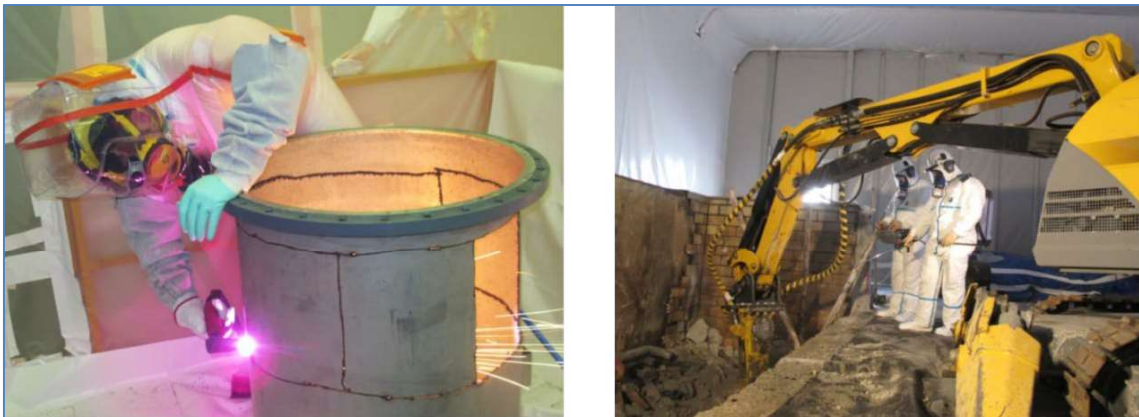
Figure 3.3.7-6. – Dismantling in confined space with PPE (left) and with a remote controlled excavator (right)
