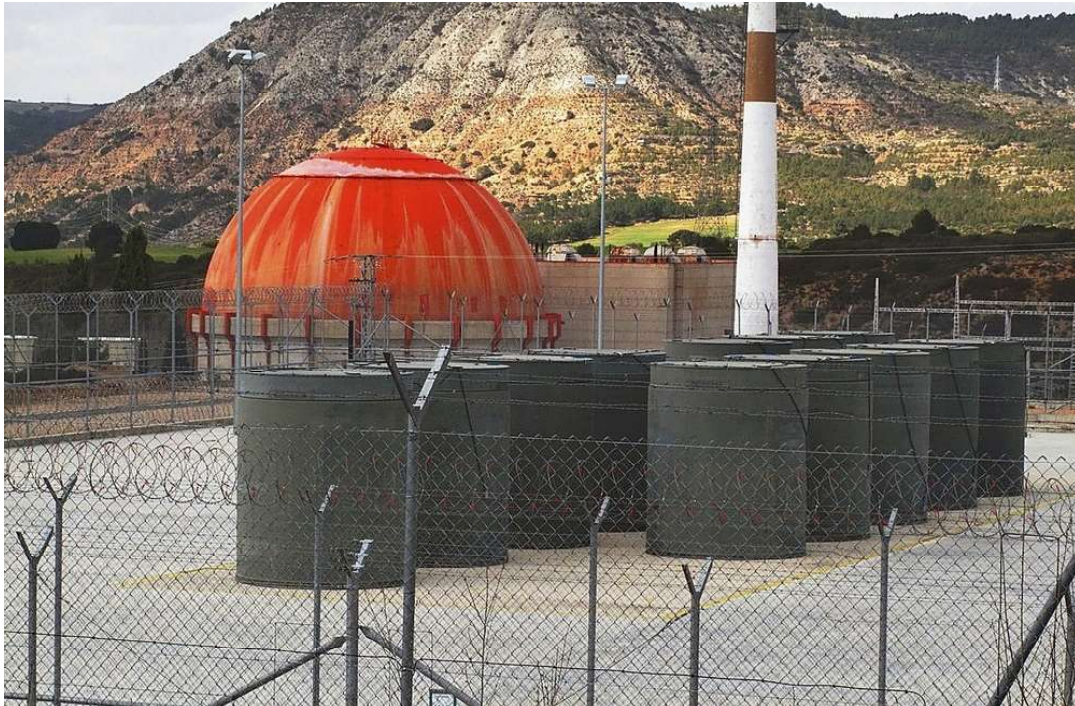
Figure 4.2-6. Outdoors spent fuel dry storage facility, José Cabrera nuclear power plant, Spain.
