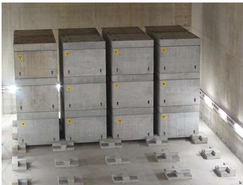
Figure 4.1-2. ILW storage at the Trawsfynydd (UK)
