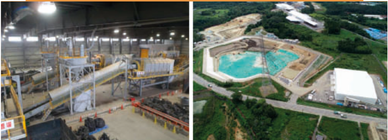
Figure 45 · Receiving and Sorting Facility (Left) and Soil Storage Facility (Right), Okuma Town, Fukushima Prefecture
